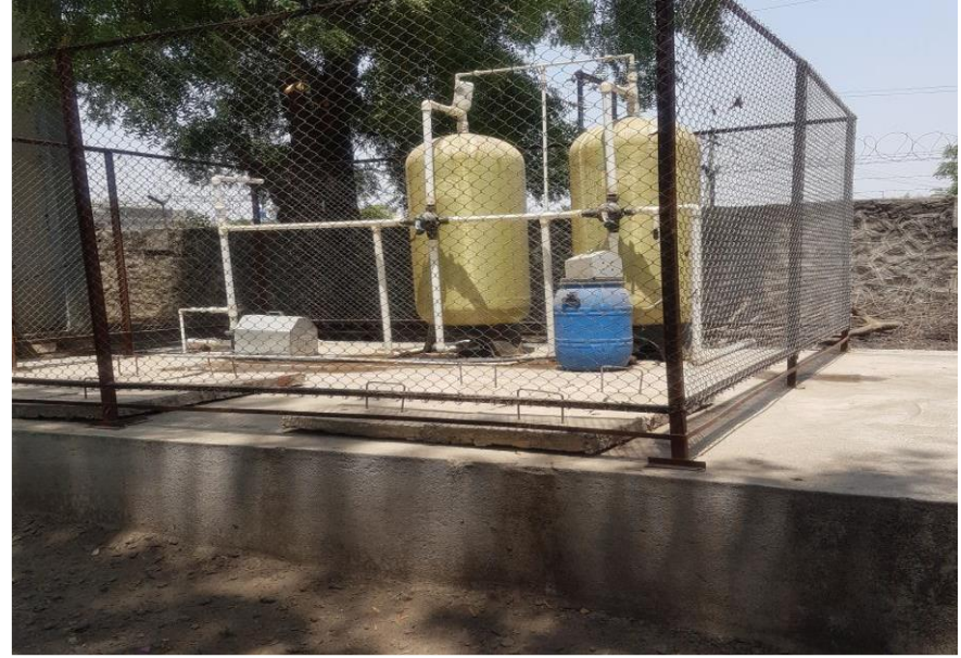
Sewage Treatment Plant ( STP )
